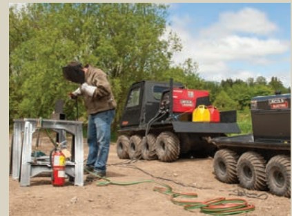
Using the multi-purpose, adaptable platform, work crews can perform a variety of tasks at remote sites.
